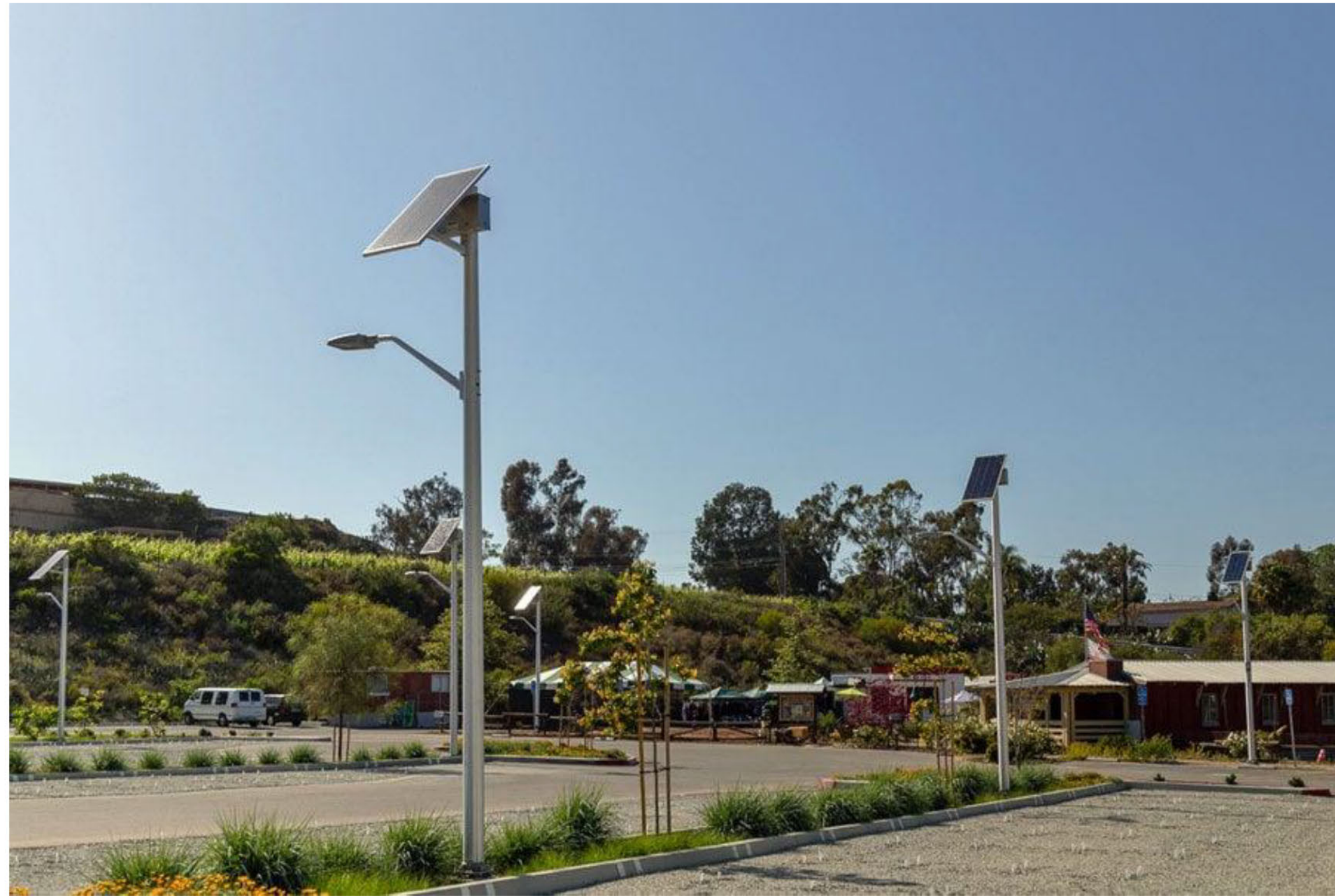
Solar parking lot lighting
